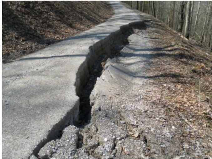
Figure 2: Slope failure resulting from a 2019 natural disaster event along Elster Road in DBNF
